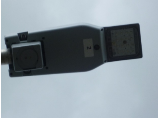
Figure 3.19 – shows a close up of one of the LED street lights in Mulberry Road.
