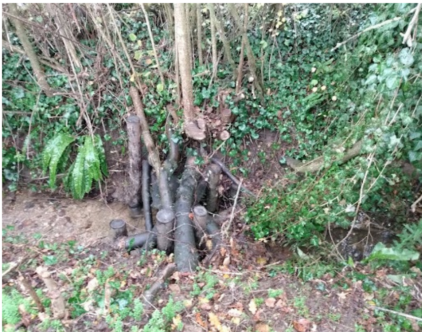
Image 11. A leaky dam was constructed along an incised tributary to slow the flow by increasing storage capacity upstream of the structure. Image credit Bristol Avon Rivers Trust
