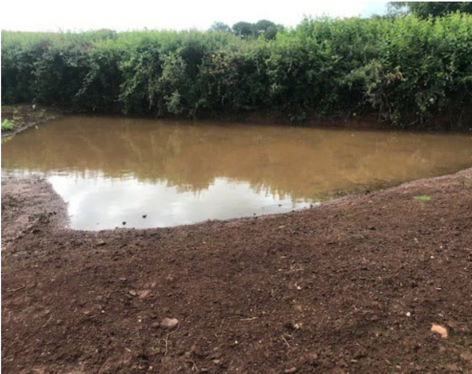
Image 10. A sediment trap designed to take water off a nearby road allows suspended sediment to settle before flowing into the downstream watercourse — image Credit Bristol Avon Rivers Trust.
