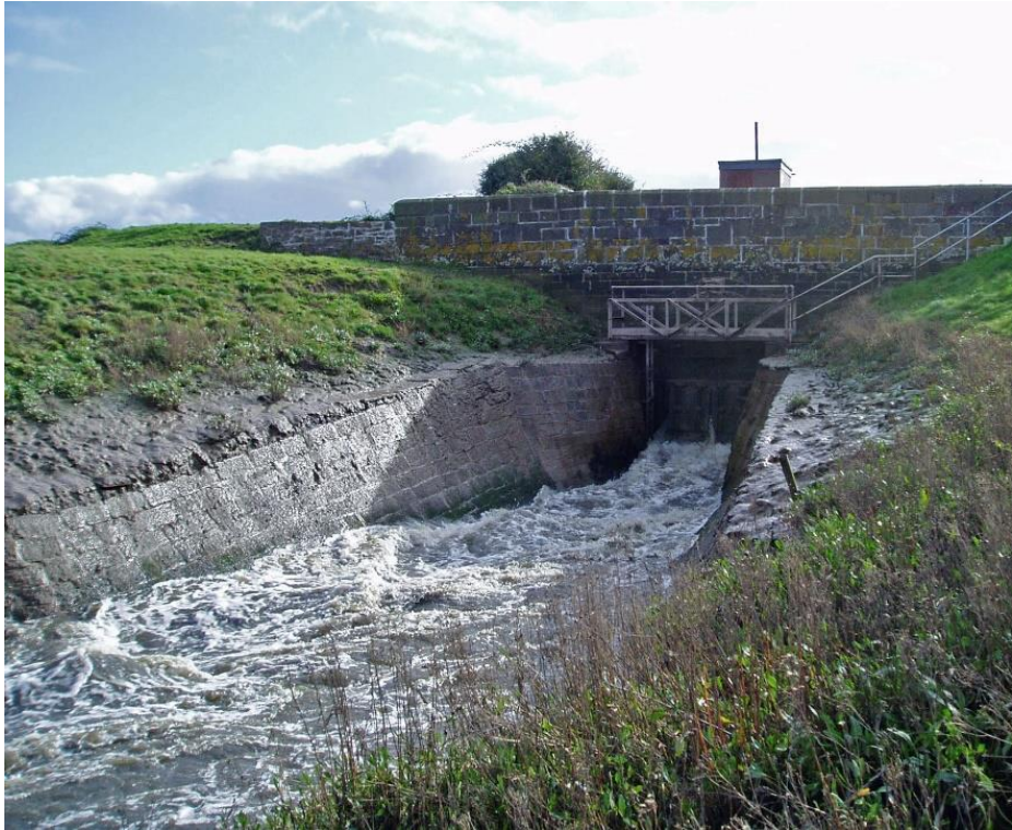
Image 11. It Shows Sampson's Sluice, where the Oldbridge River meets the flood defences along the coast. Sluices and flaps like these ensure a continuous line of protection along the coast.
