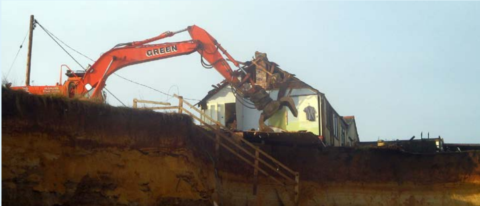
Figure 13: A property at risk of coastal erosion being demolished (image courtesy of North Norfolk District Council).
