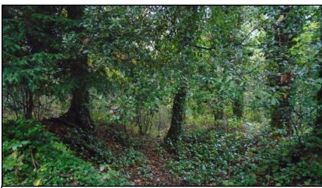
Figure 19: Trees and vegetation along ramparts. Roots here are causing damage to the rampart material
